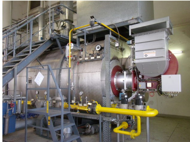
The new combi-burner for energy.
