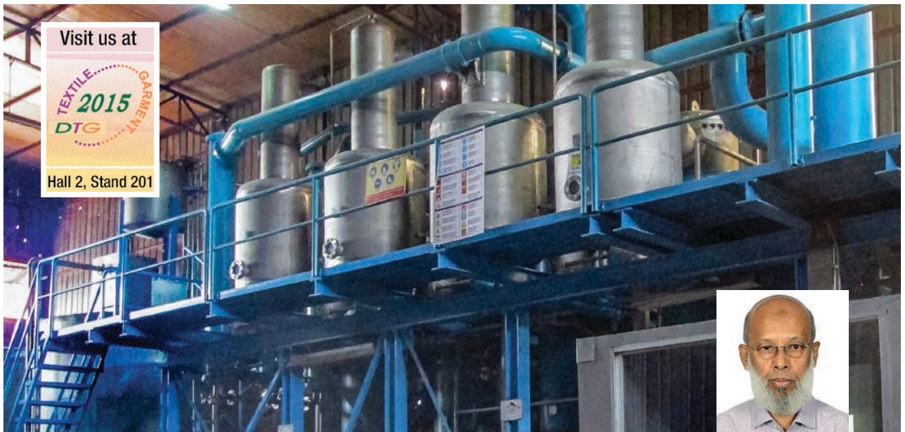
Caustic recovery plant in Dhaka, Bangladesh
