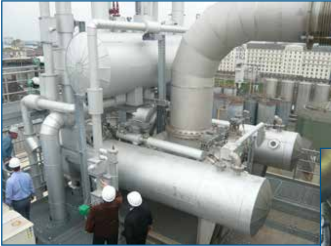
Ice condensation block completely installed at site
